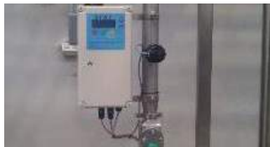
Wall mount connection on a control panel of a bottled water plant (Australia). Series TH387.
