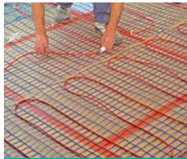
Heating cables connection.
