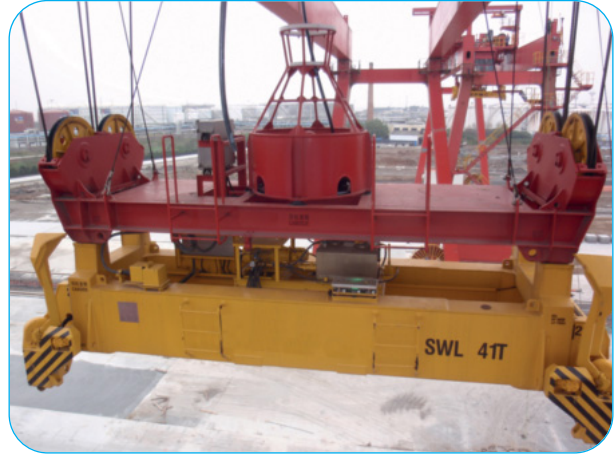
spreader power cables
