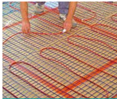
Heating cables connection.
